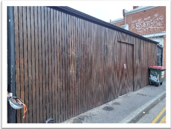
Image 8 - Graffiti noted on Field Street - Gauchos Restaurant – after.
