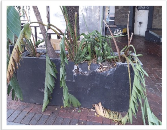
Image 26 - Planter box requiring maintenance.
