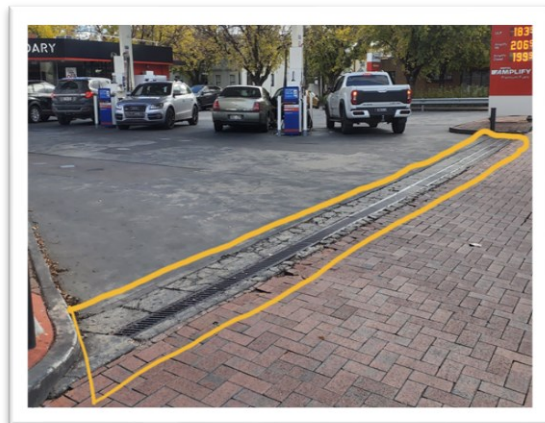
Image 53 - Damaged infrastructure 131 O'Connell Street
