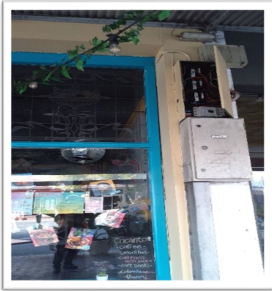
Image 15 - Missing fuse box cover
