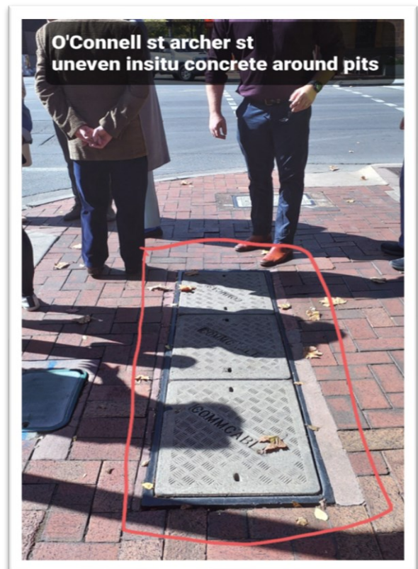
Image 37 - Area of paving requiring maintenance
