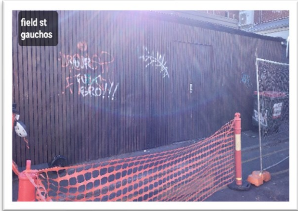
Image 7 - Graffiti noted on Field Street - Gauchos Restaurant – before.
