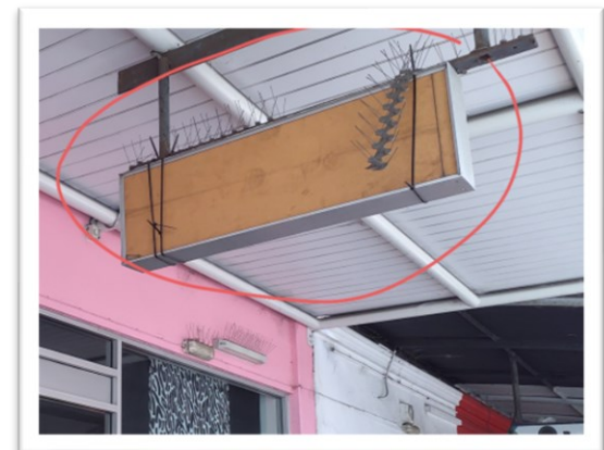
Image 55 - Anti-bird device not installed correctly.
