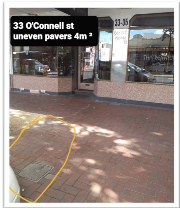
Image 36 - Area of paving requiring maintenance
