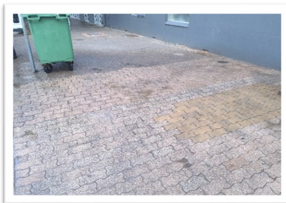
Image 32 - Progress shot of deep cleaning showing grime removal in process - 22 O'Connell Street
