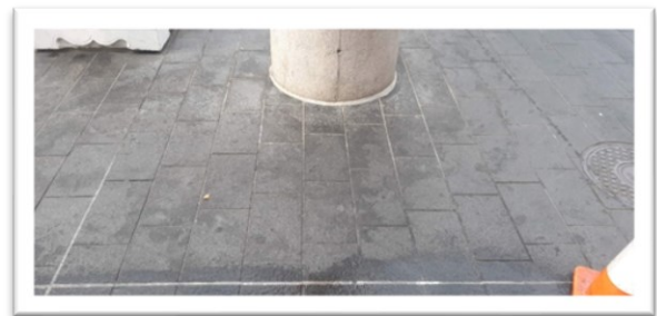
Image 1 - Before - Stains and chewing gum - Moonta Street entrance
