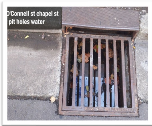
Image 52 - Catch pit holding water.
