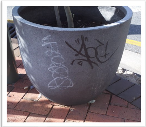
Image 13 – Graffiti observed on a pot plant – corner of Gouger Street and Mill Street
