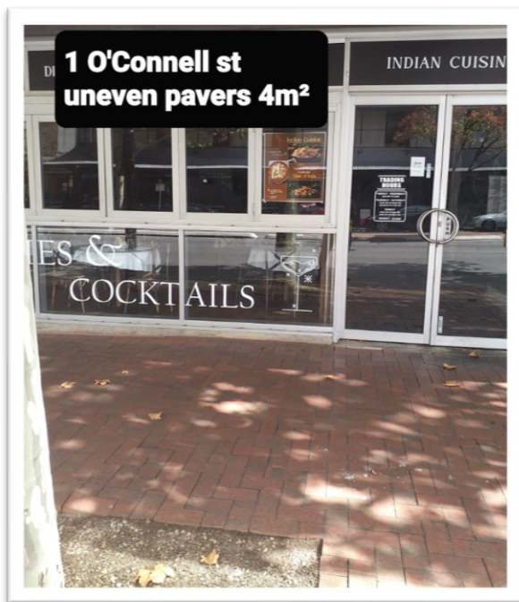
Image 35 - Area of paving requiring maintenance
